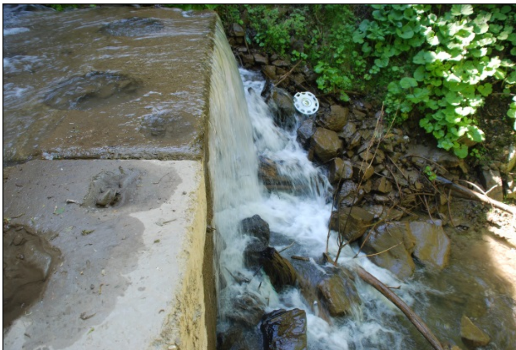
Figure 6: Concrete threshold of three m height, with no fish ladder on the upper Vişeu River.
